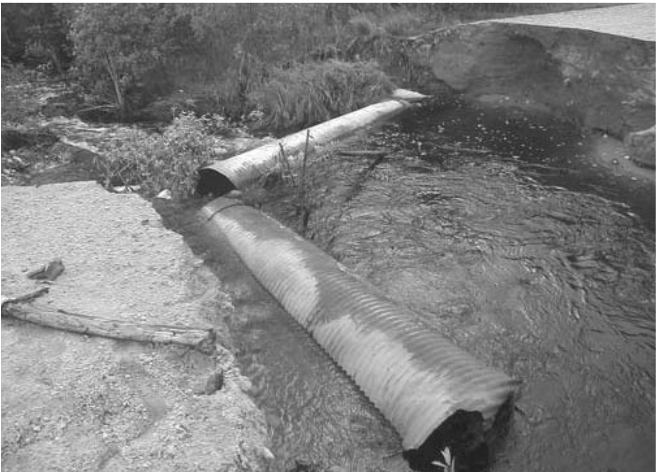
Culverts were washed out
